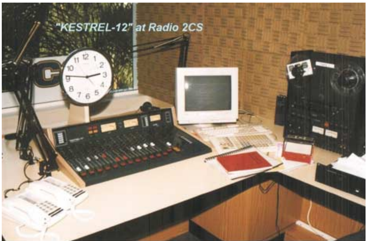
"Kestrel-12" Mixer installed at Radio 2 CS Coffs Harbour NSW
